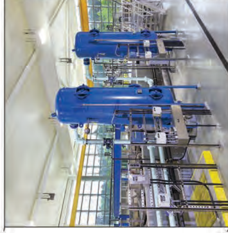
CLEAN AND SIMPLE PROCESS AREA
