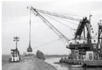
In this Feb. 15 photo, a load of rocks is dropped to patch a crater as repairs are made on the Tyler Island levee near Isleton. RICH PEDRONCELLI/AP
