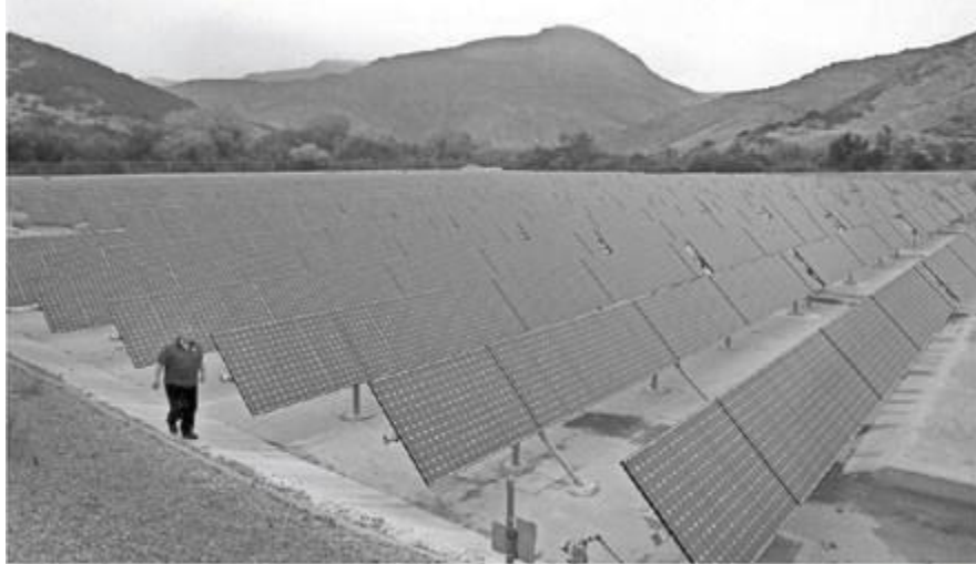
Santos Marquez, a laboratory supervisor for the Thousand Oaks Public Works Department, looks over the solar panels at the Hill Canyon Wastewater Treatment Plant. They installed 2,783 panels at the facility to create half of the plant's power. JUAN CARLO/THE STAR
