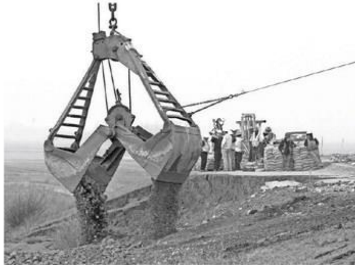
In this Feb. 15 photo, a load of rocks is dropped to patch a crater as repairs are made on the Tyler Island levee near Isleton. RICH PEDRONCELLI/AP
