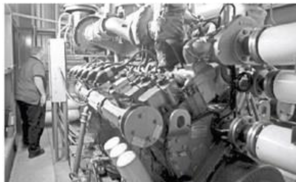
Santos Marquez, a laboratory supervisor for the Thousand Oaks Public Works Department, checks on the engine that makes power through the methane gas they collect at the Hill Canyon Wastewater Treatment Plant. JUAN CARLO/THE STAR
