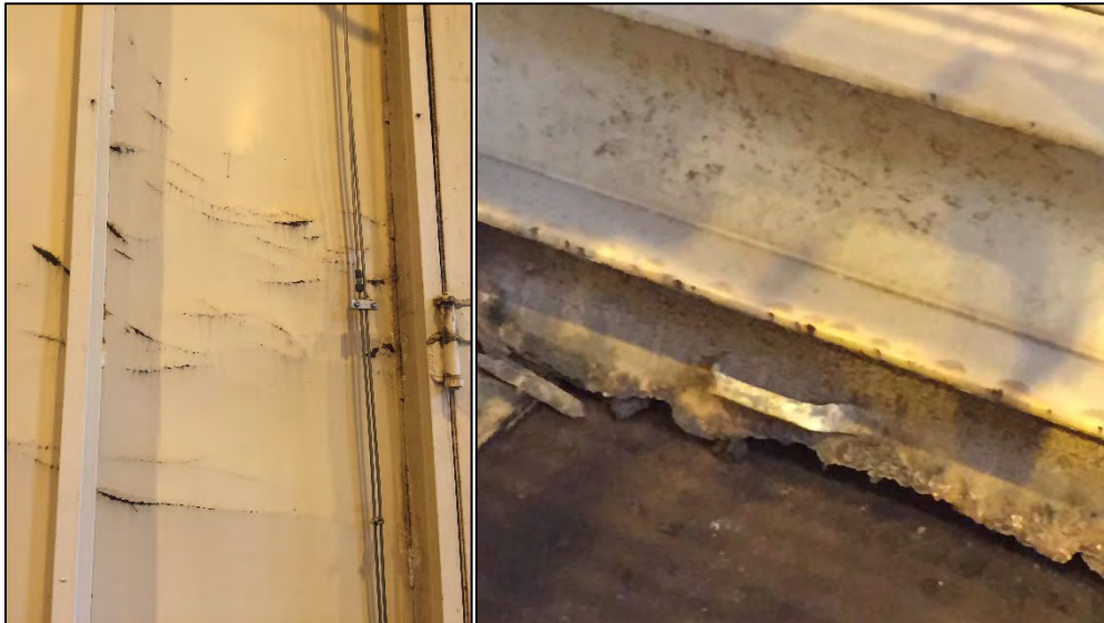
Figure 9 Exterior Damage and Corrosion in Bulk Amendment Bin
