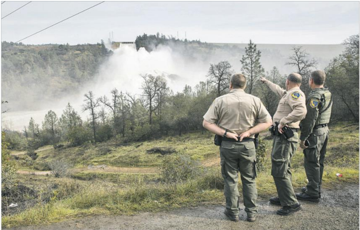
WARDENS from the California Department of Fish and Wildlife watch as water from Lake Oroville cascades out of the reservoir's damaged primary spillway at 100,000 cubic feet per second. More than 100,000 people were evacuated downstream of the state's second-largest — and nation's tallest — dam Sunday. BRIAN VAN DER BRUG LOS ANGELES TIMES
