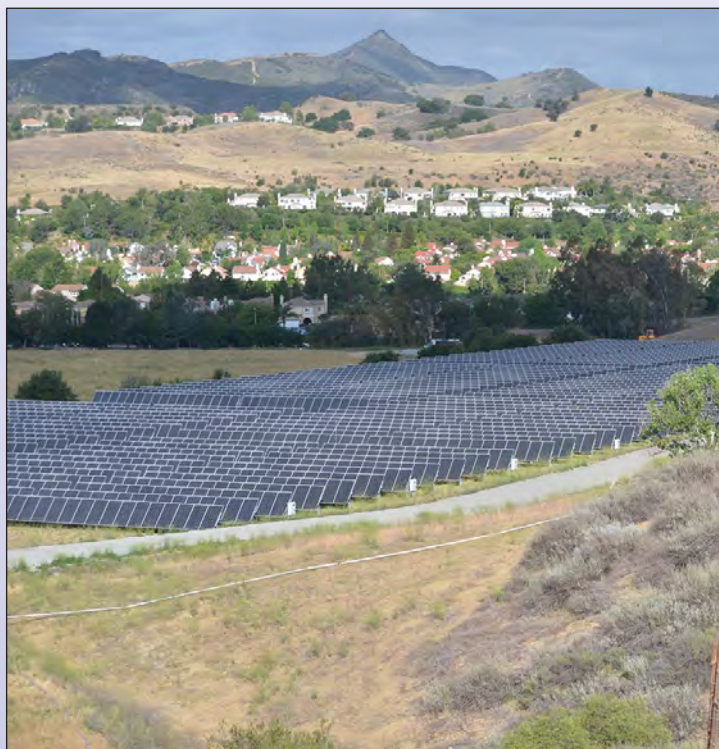
One megawatt solar power facility used to pump recycled water in Calabasas, CA.
