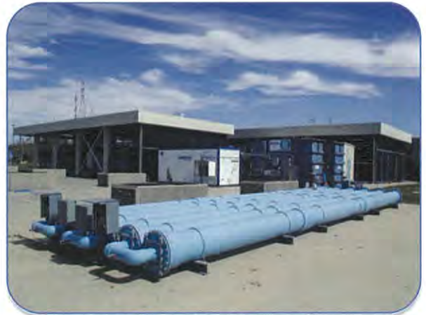
San Diego Advanced Water Demonstration Facility
