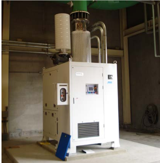
Figure 4.3 Typical Turbo Blower Installation
