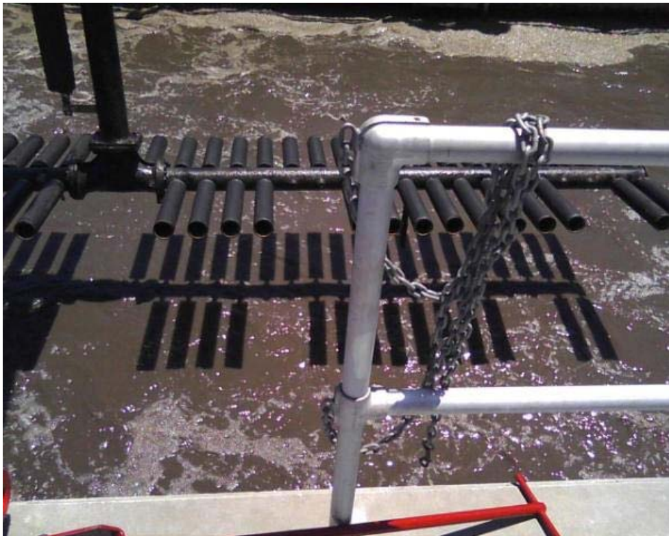
Pictures 8 (top) and 9 (bottom) showing swing arms with fine pore tube diffusers. Diffusers removed in pairs to clear hand rails when the swing is fully retracted to the wall.
