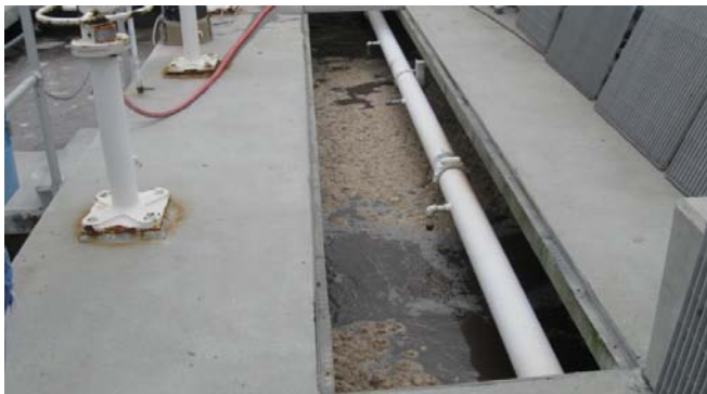
Figure 4.9 Un-aerated Segment of Mixed Liquor Channel
