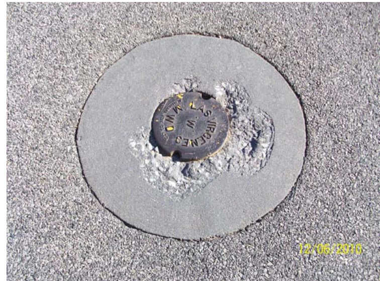
Existing Valve Can on Park Capri
