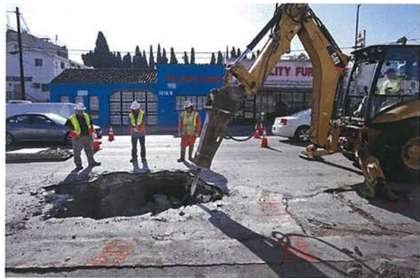
DWP workers break through Alvarado Street to access a broken water pipe. (Al Seib / Los Angeles Times)
