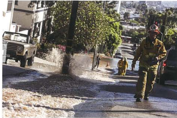
DWP workers break through Alvarado Street to access a broken water pipe. (Al Seib / Los Angeles Times)
