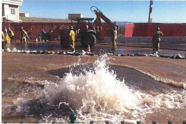
Firefighters and workers clear mud and water at Pauley Pavilion after a major water trunk break. (Jabin Botsford / Los Angeles Times)
