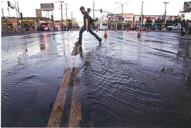
A firefighter follows a water pipe break on Sunset Boulevard. (Emily Rhyne / Los Angeles Times)
