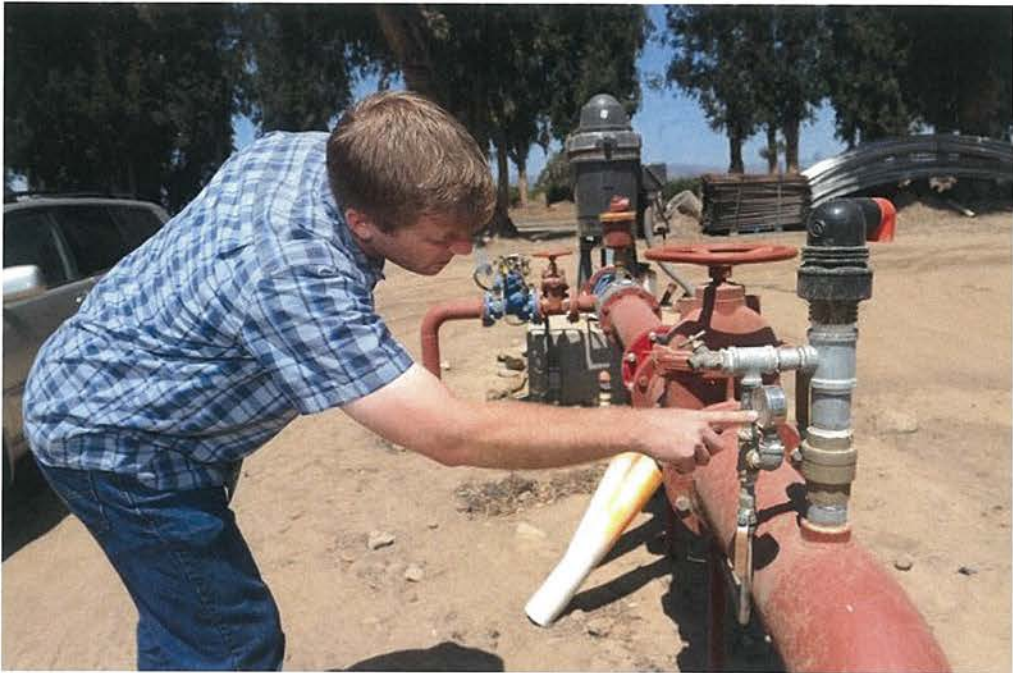
ROB VARELA/THE STAR Jason Vis checks a pressure gauge on a pump at Lloyd-Butler Farms near Saticoy.
