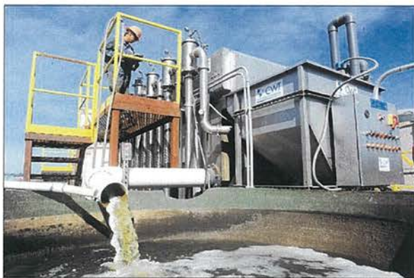
Mark Albillar, operator, at Southern California Waste Water in Santa Paula checks the PH levels on the GEM system.
