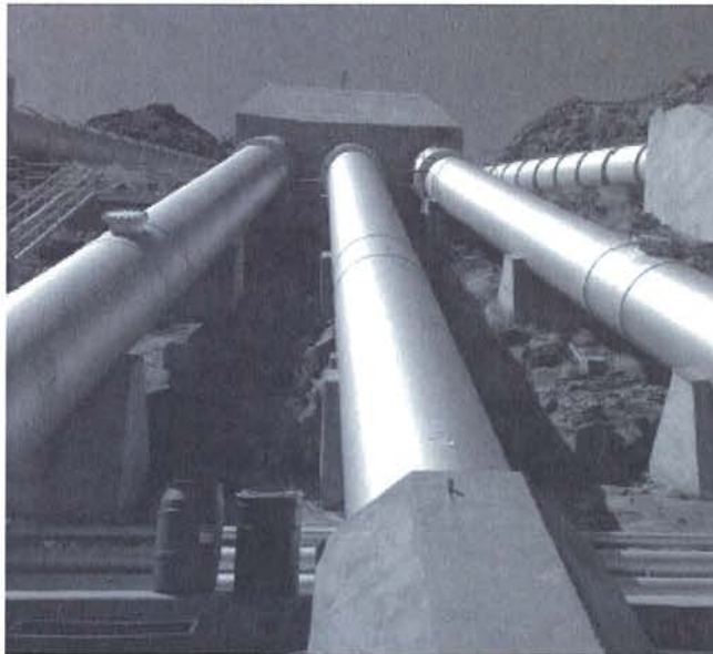
The giant pipes at the Gene Pumping Plant.
