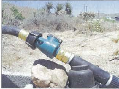
Use Teflon tape for plumbing to repair any leaks or seeps in your drip system couplers. Maureen Gilmer/MCT Yardsmart
