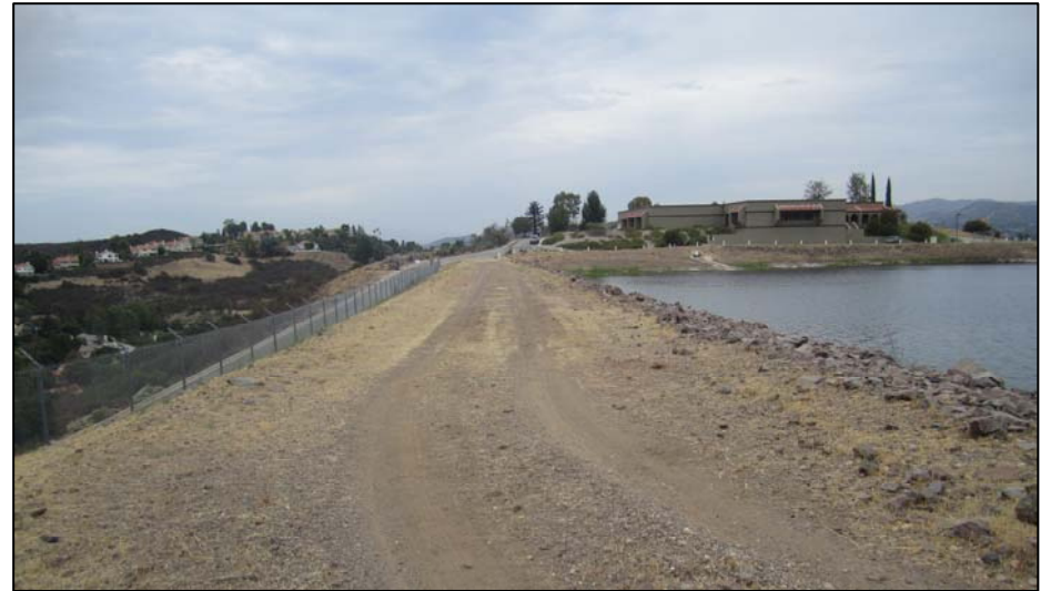
Photo 2. View looking north across the dirt access road and western reservoir dam embankment. Las Virgenes Reservoir is on the right.
