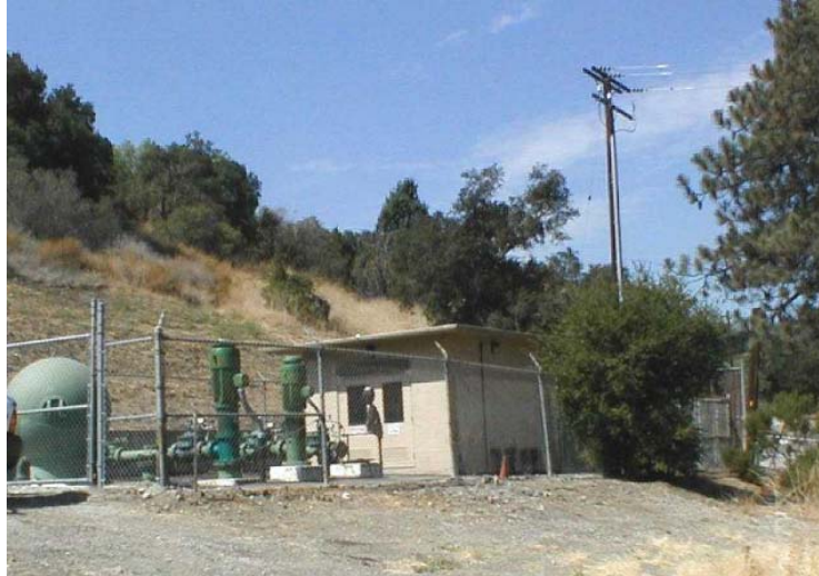
Figure 9—Warner Pump Station
