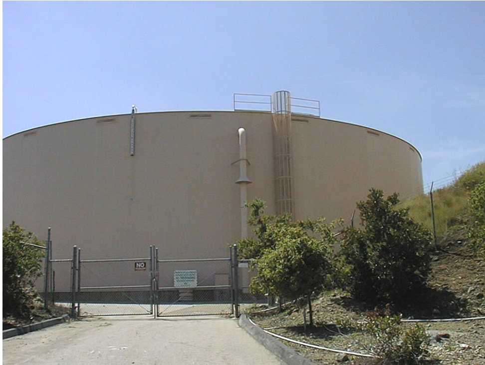
Figure 26—Indian Hills Tank
