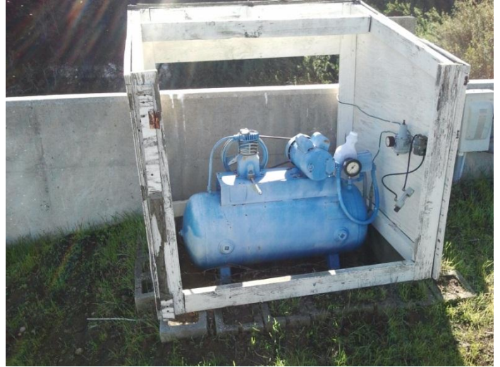
Figure 20—Reservoir 1 air compressor
