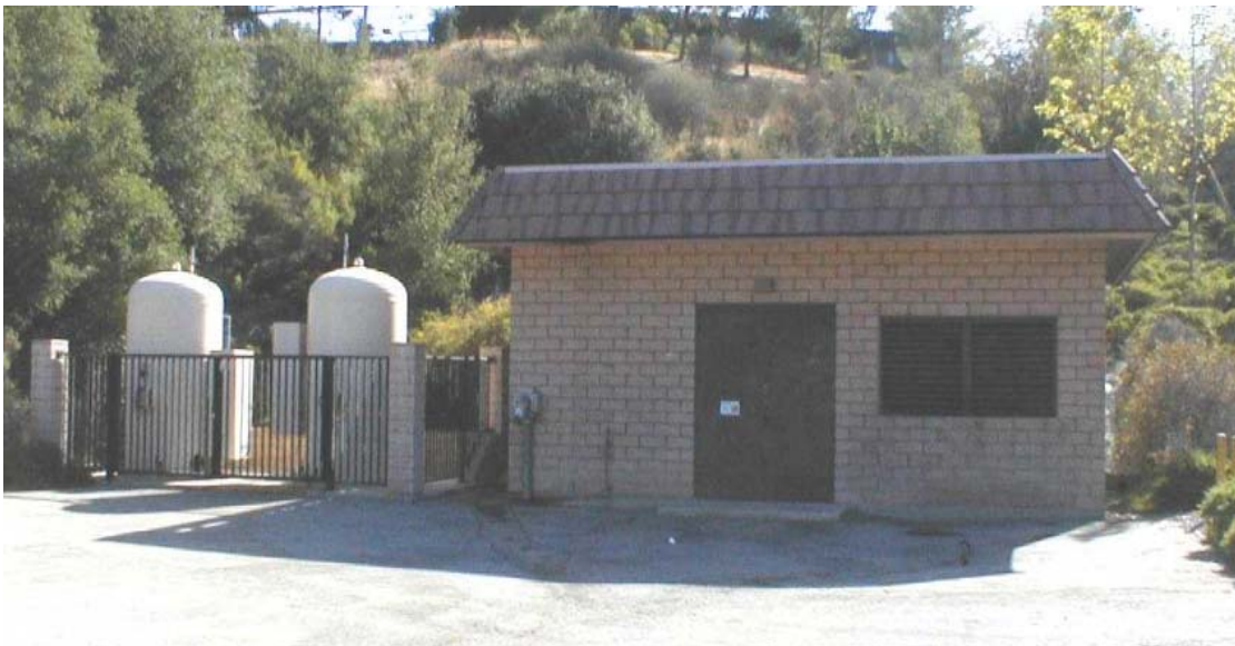
Figure 24—Seminole Pump Station
