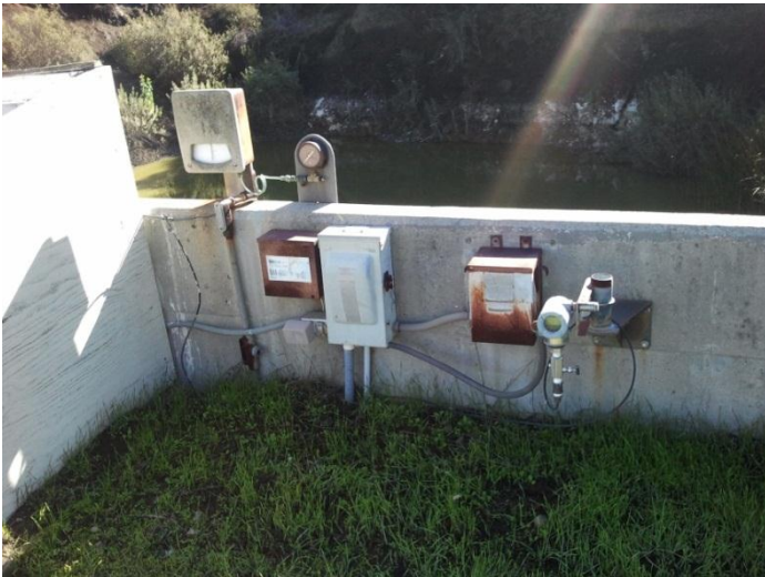
Figure 21—Reservoir 1 air compressor electrical outlets. Will use to power the Tapia repeater
