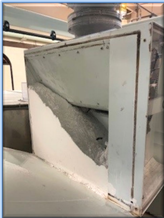
DE leak inside precoat bins (above left)
