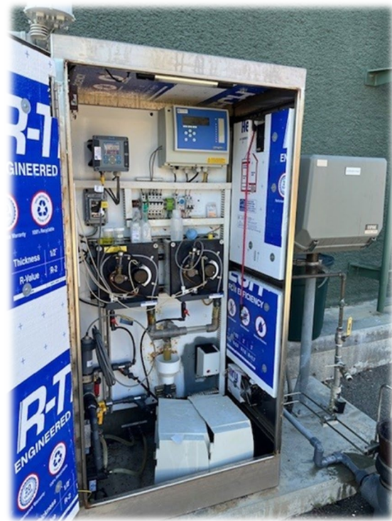
Torchwood Tank Analyzer Cabinet - After
