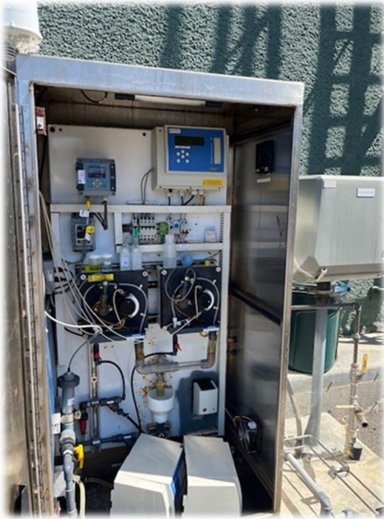
Torchwood Tank Analyzer Cabinet - Before
