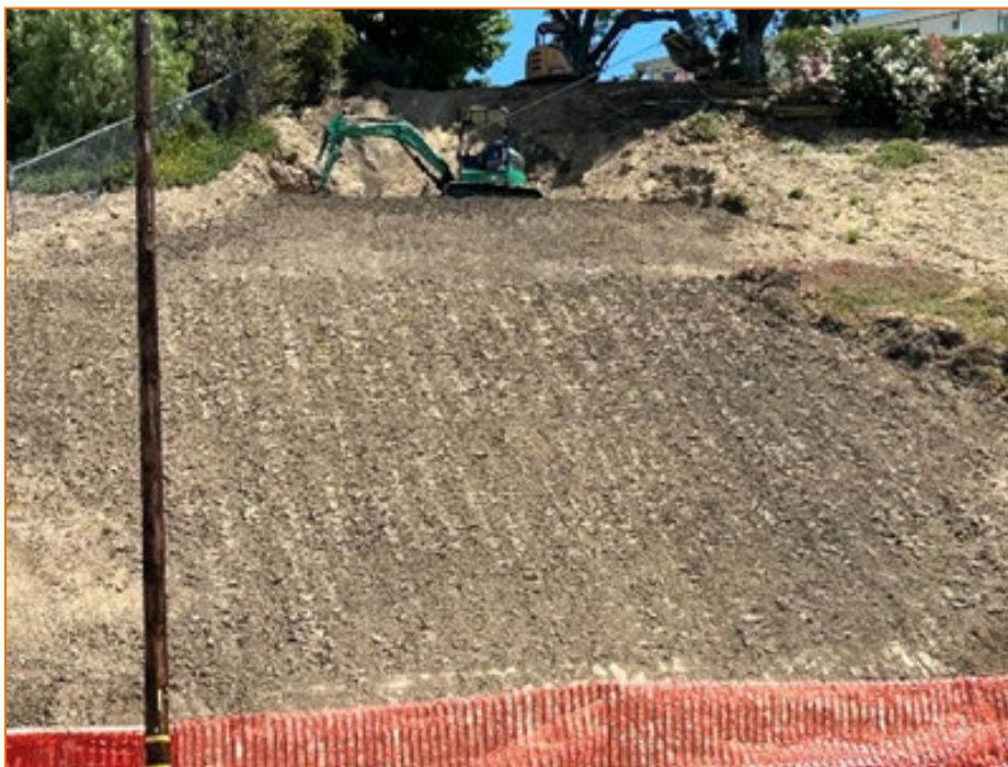
(photo left) View of the slope repair from Thousand Oaks Blvd. looking up towards homes on Parkmore.
