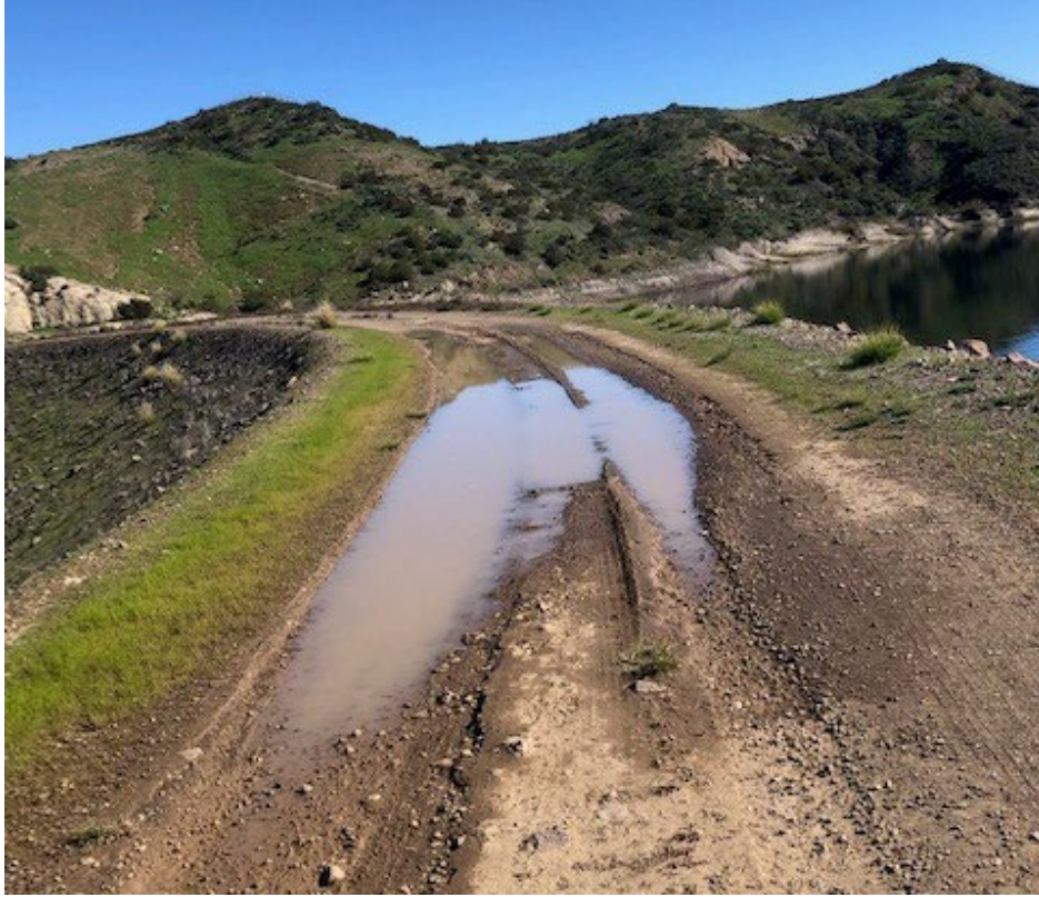
Figure 2 - Access road following rain.
