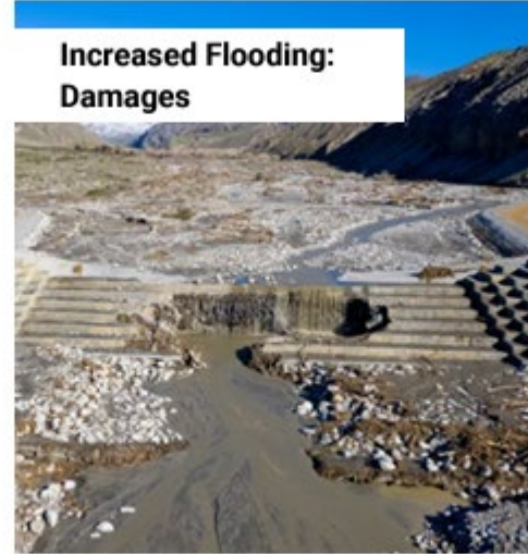
Flood damages at the Whitewater River near the Colorado River Aqueduct.
