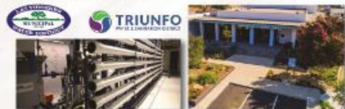
Opened in 2020, the Pure Water Demonstration Facility provides the opportunity for JPA customers to learn first hand how the advanced purification process works.
