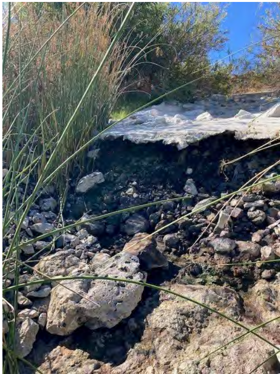
Photo 6 – Undermined Spillway Riprap
