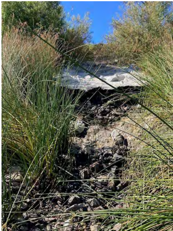
Photo 4 – Undermined Spillway Riprap
