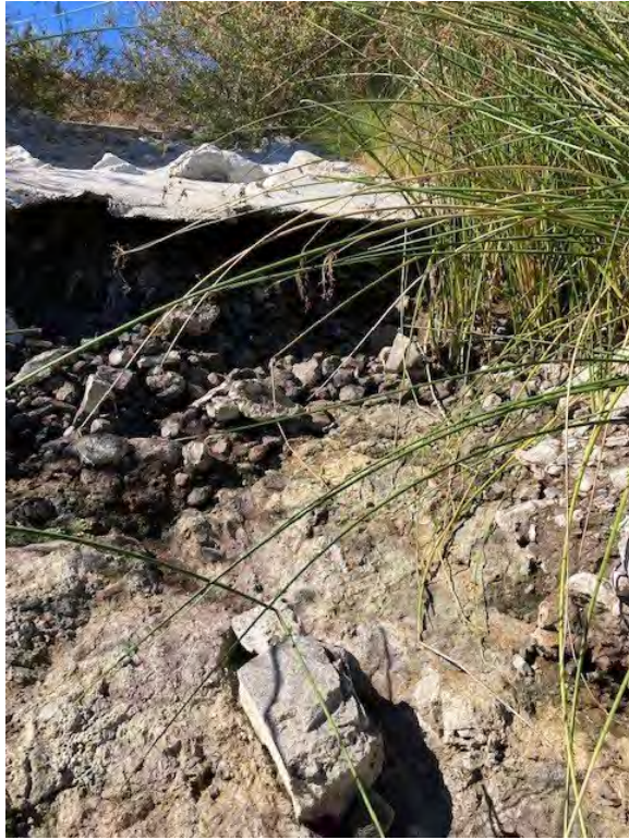
Photo 5 – Undermined Spillway Riprap
