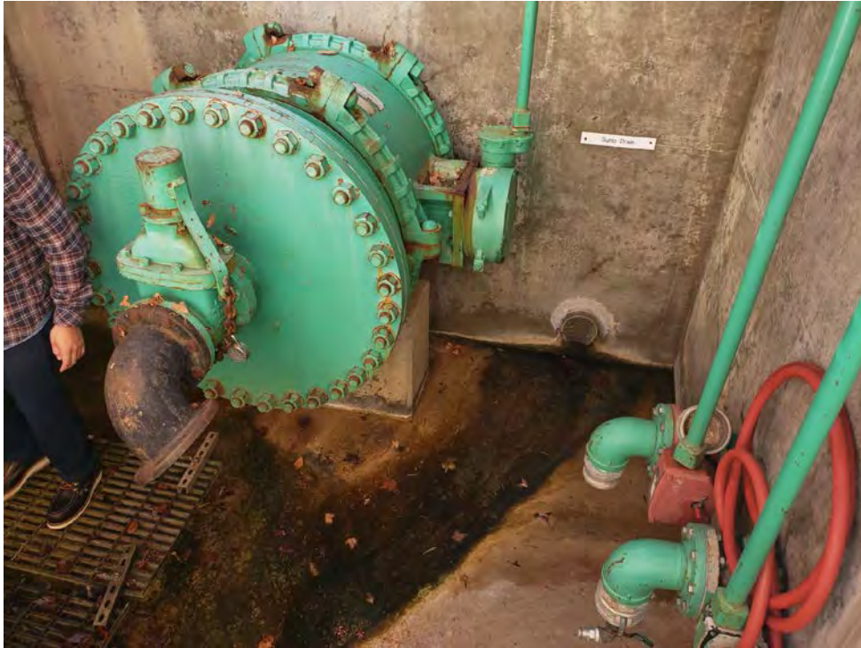
Corroded items in the downstream valve vault recommended to be cleaned and re-coated.
