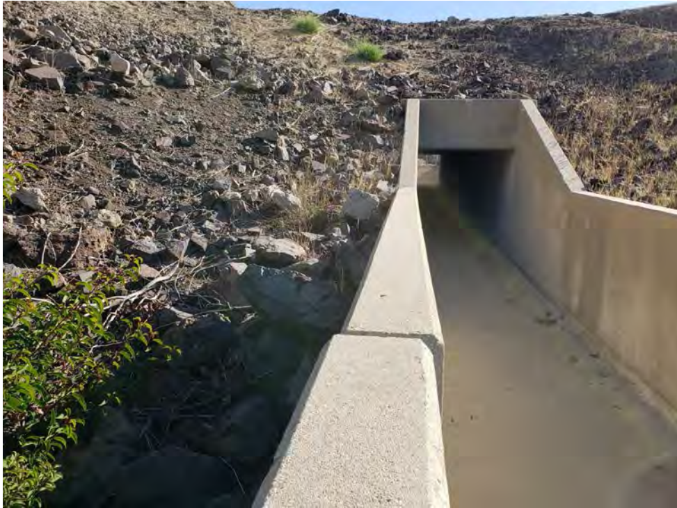
The misalignment to the spillway wall joints appeared unchanged.
