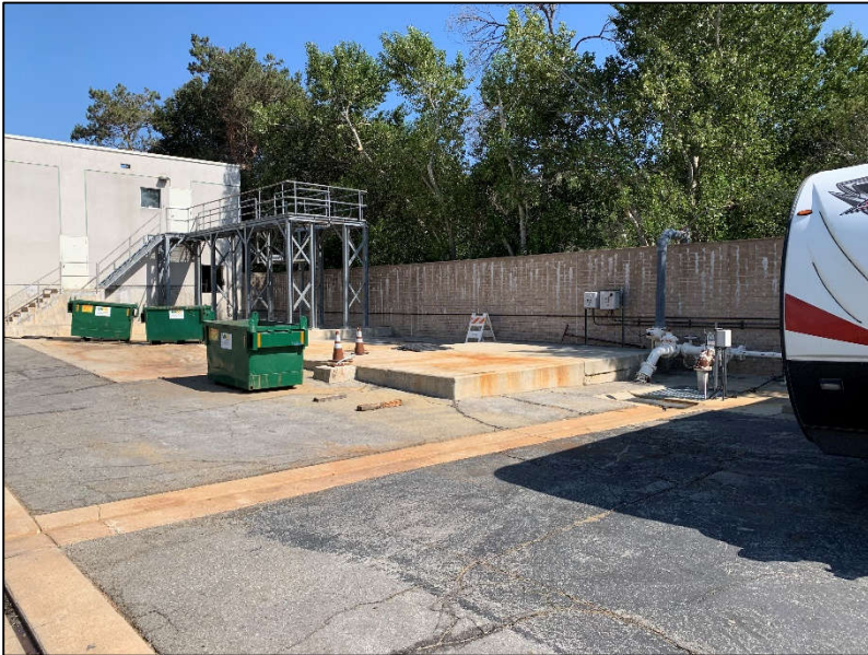
c. Battery storage system site at Tapia Water Reclamation Facility
