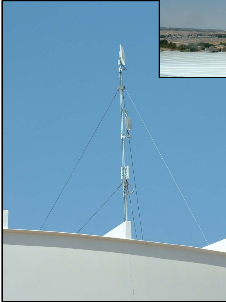
Figure 3-3 Tank Mounted Antenna Mast with Integrated Transceiver and Antenna
