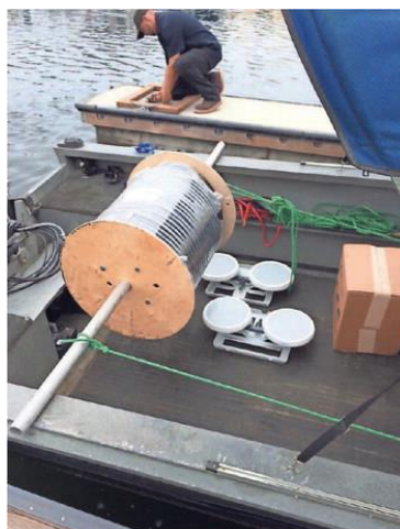
A worker begins to install aerators at Channel Islands Harbor in Oxnard. Water quality started decreasing in June in an apparent algae bloom. COURTESY OF CITY OF OXNARD
