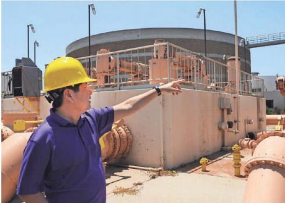
Thien Ng, the city of Oxnard's assistant public works director, stands in front of an old water pump at the city's sewer plant. The facility is in need of major improvements. PHOTOS BY CHUCK KIRMAN/THE STAR
