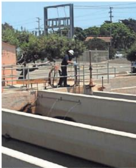
This is the chlorine contact tank at Oxnard's
