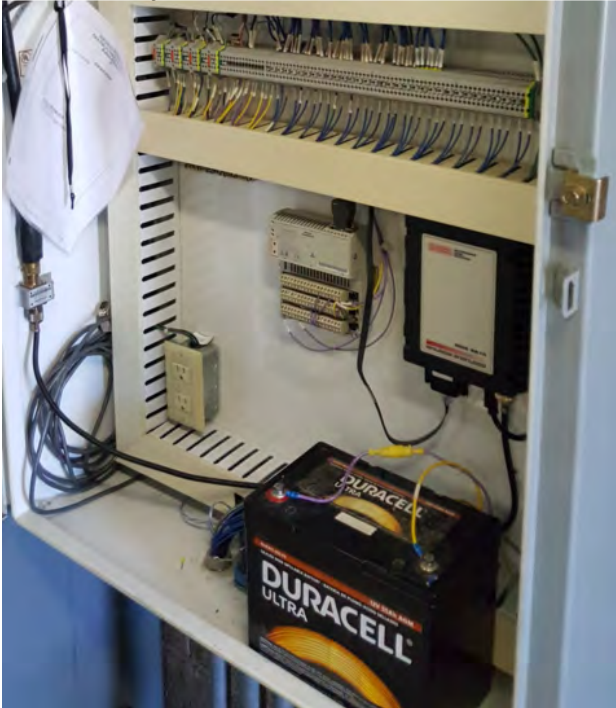
Figure 2-2 – Water Operations panel with standard battery backup
