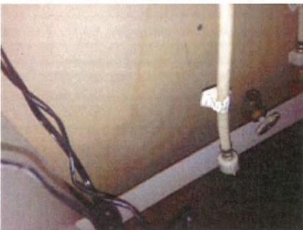
Moisture on wall, behind cabinet.JPG 58K
