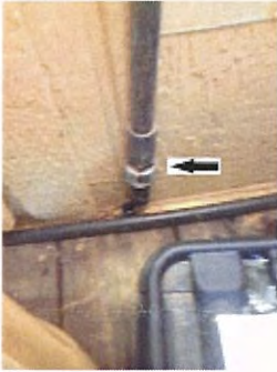
Snapped pipe, exterior.JPG 74K
